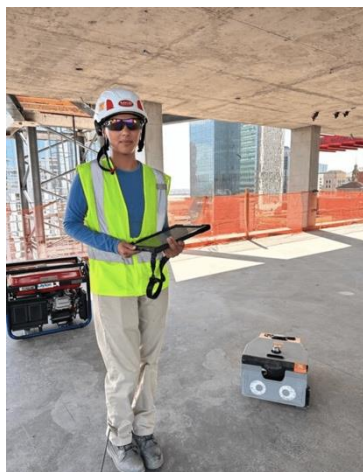
Alezet Valerio on the construction job in Phoenix with the robot that assists with site layout. PHOTO: BASHAR ALAOUDI/DUSTY ROBOTICS
